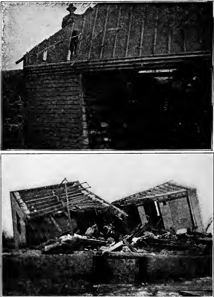
FIG. 472. — Destruction by tornadoes. Upper view (W. L. Ikenberry) shows laths driven into house at Mt. Morris, Ill. Lower view (A. W. Dunwiddie) shows house turned upside down near Janesville, Wisconsin.
